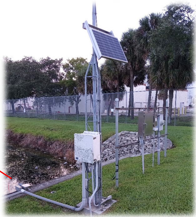
Water Level Monitoring Device
